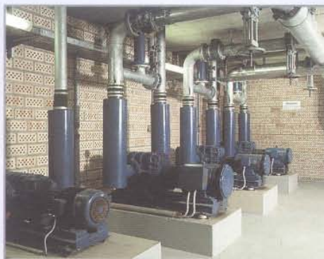
Water supply facilities
